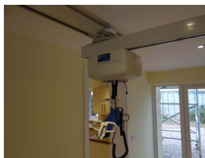
➤ Therapy Room: OT200 compact Ceiling Hoist on XY to XY frame for full-room coverage
