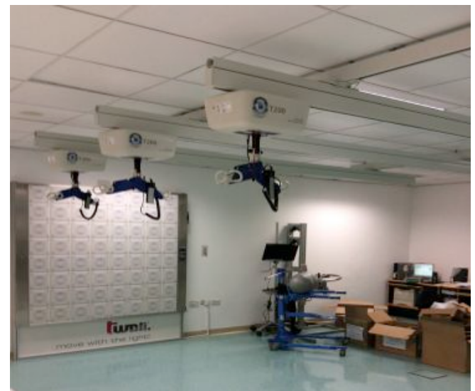
The Occupational and Rehabilitation Departments opted for multiple H systems to allow several patients to be assessed at the same time using the OpeMed walking harness
