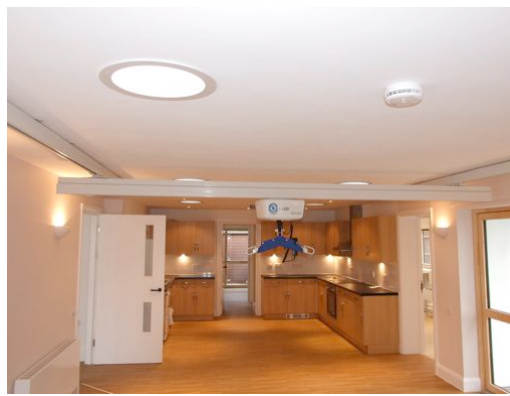
OT200 on H System in Lounge/Kitchen
