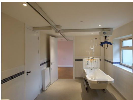
OT200 over OpeMed 1700 Bath. Note the turntables bringing the track in from the bedroom over the bath & continuing into the next bedroom
